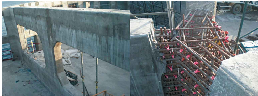
Figure 4 Detailed view of the central shear wall and panel joint between the curved shear walls
