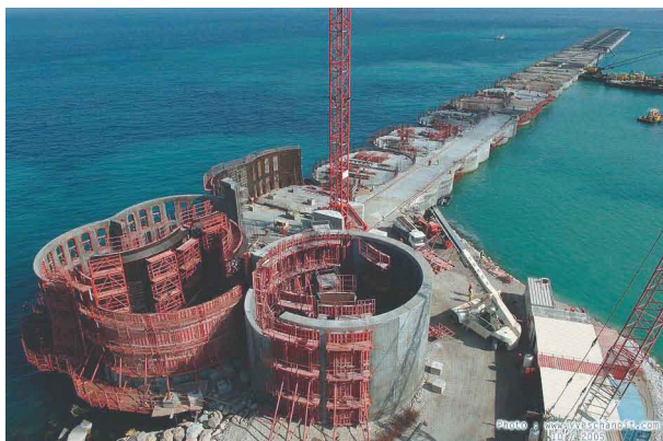
Figure 2 Top view of a box girder during building of the superstructure shear walls
