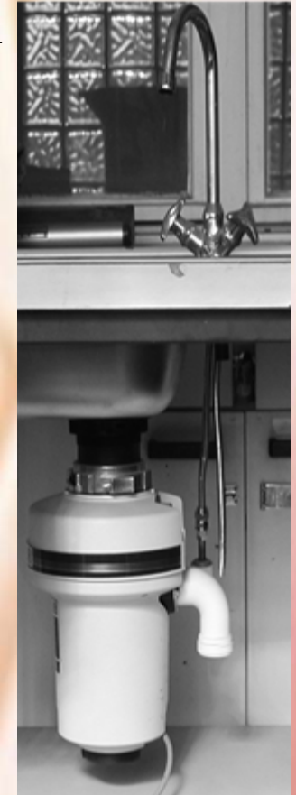
Wash basin + Garbage grinder
