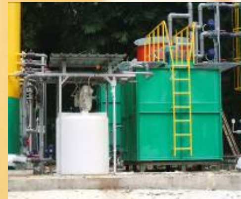
Food waste plant for biogas production
