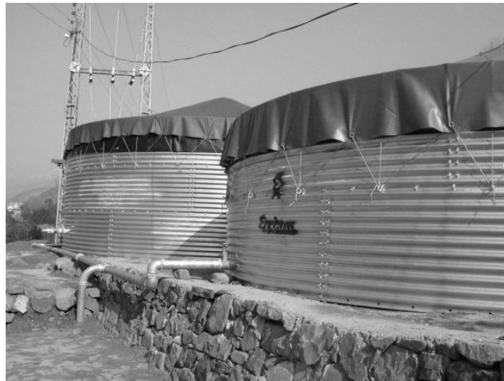
Figure 3: Emergency batch sedimentation tanks used in Gahri Dupatta.
