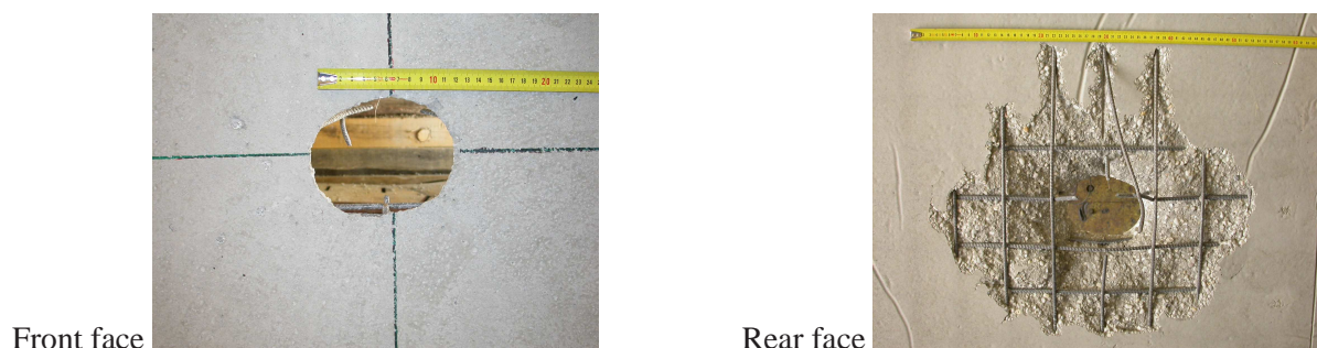
Fig. 3: Damage of the reinforced concrete slab after test n°1 ( V_0 = 107.5 m/s)
