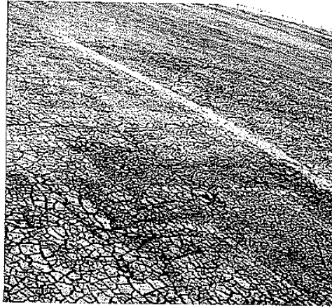
Figure 2: Hairline cracking on bituminous concrete facing dam leading to score 6 given to the watertightness component protection function
