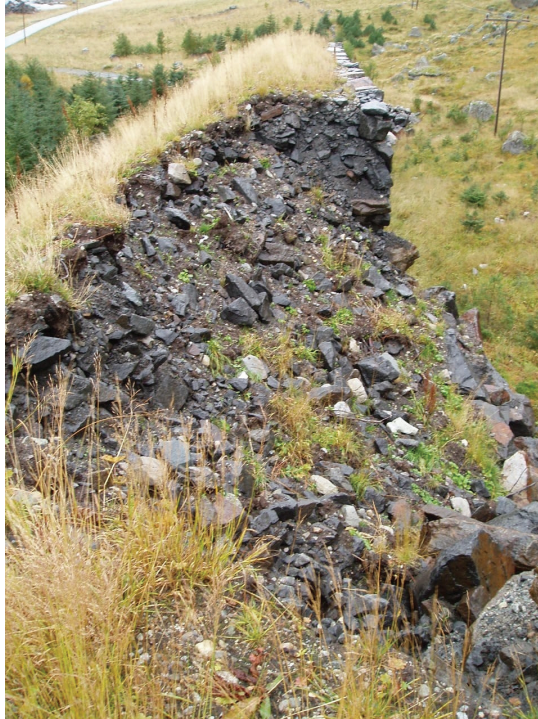
Figure 15.2: Failure in an avalanche retaining dam. The dam height is 8 m. (Photo: Karstein Lied.)
