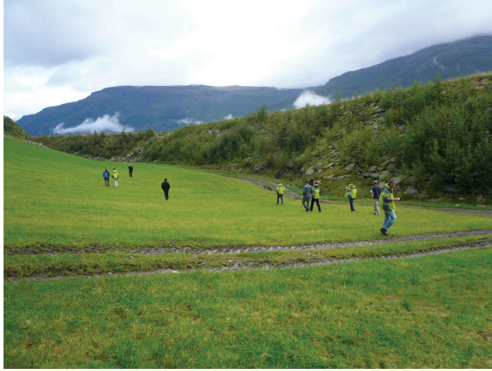
Figure 15.5: A catching dam for wet snow avalanches and debris flows. Dry wall with backfill of earth materials, height 12 m, inclination 1:1. Ullensvang, Norway. (Photo: Karstein Lied.)
