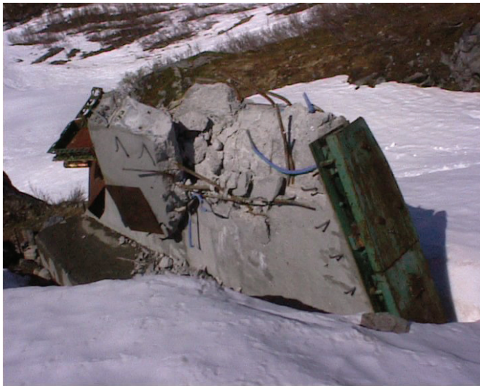
Figure 13.1: Damage caused by an impact of solid debris at the NGI test site Ryggfonn (photo: NGI; Avalanche event 20000217 13:55).
