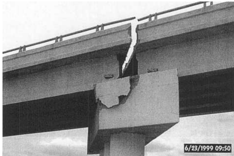
Figure 1. Damage of a skew bridge after the Tehuacan 1999 Mexico earthquake [6].
