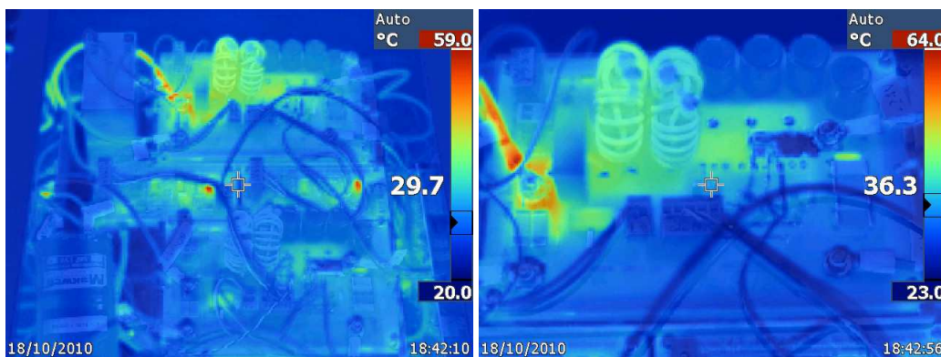
Figure 8. Temperature of the power converters after 1h operation at rating load
