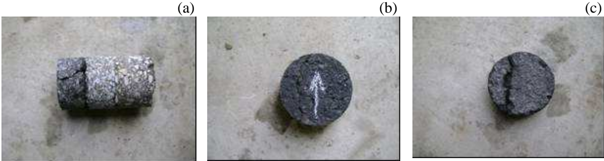
Figure4: Core sample taken at longitudinal crack level. (a) The first interface is detached whereas the first layer is cracked straight down. (b) View from above the wearing course. (c) View from below the wearing course.
