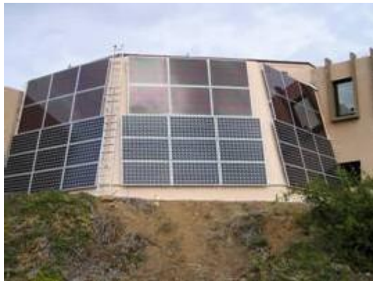
Figure 8: The frontage PV system on the Vignola laboratory walls.
