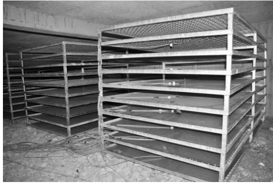
Figure 3 : Instrumented multi-layer rack in the crawl space.
