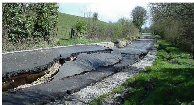
Figure 1. Example of a damage induced by a landslide triggering in the Pays d'Auge plateau (Source: TP-Geo)
