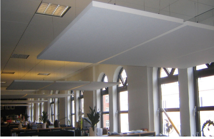
Figure 3. Free hanging absorbing units above workplaces
