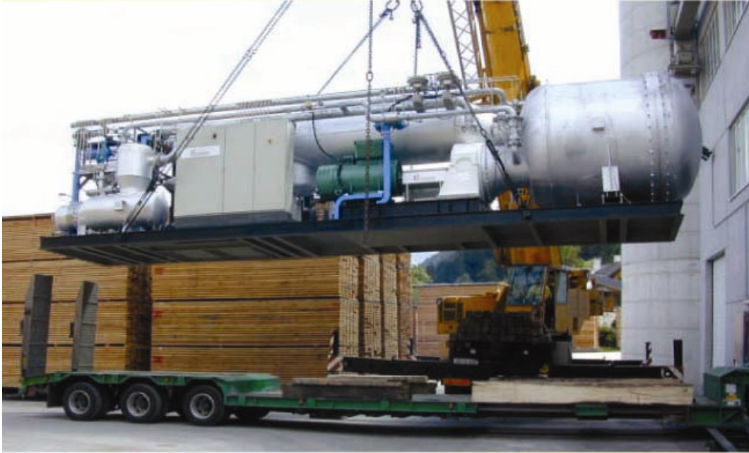
Fig. 9 Overview of the Whole Module of the Biomass-Fired ORC Plant (from Ref. 25)
