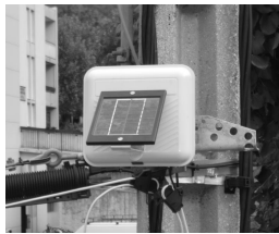
Figure 6: A solar powered gateway.
