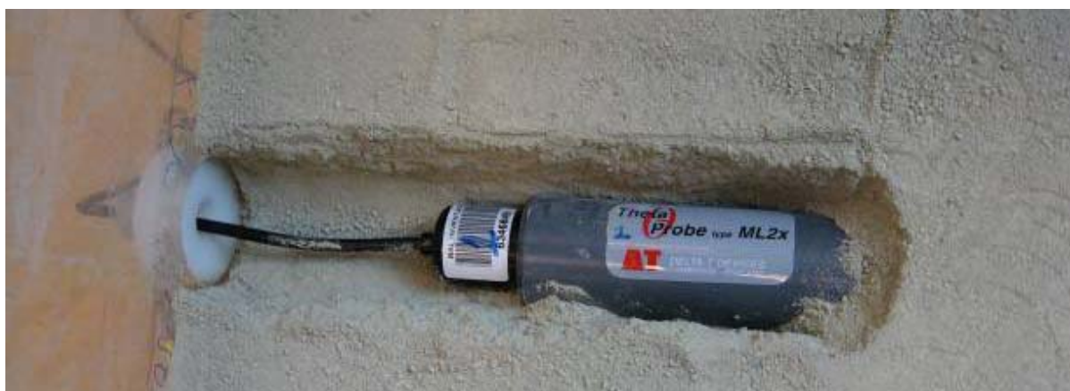
Fig. 4. Installation of the ThetaProbe (TP) sensors
