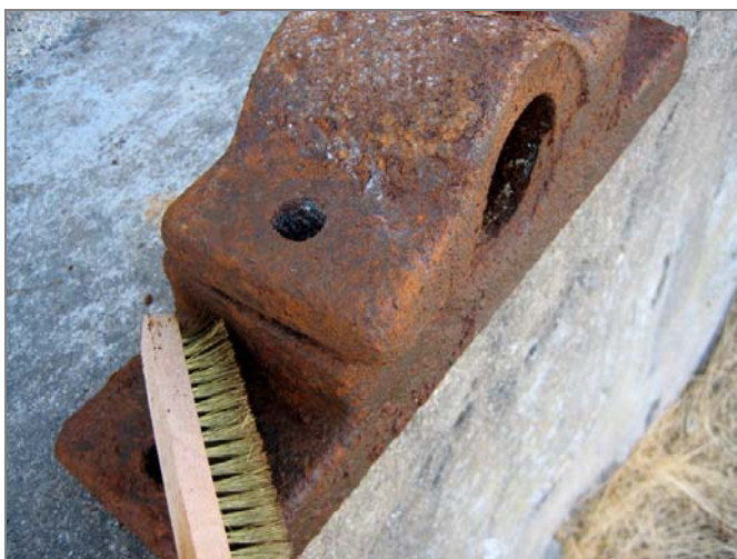
Figure 20: Photograph of unused bearing (2007)
