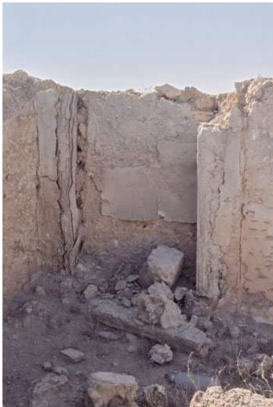
Figure 6. Example of a door blocked with mudbrick.
