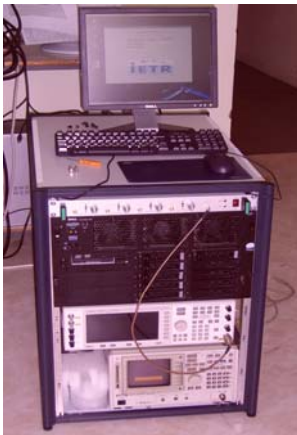
Figure 3: Receiving and acquisition system.
