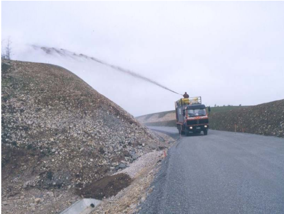
Figure 2. Hydroseeding technique particularly adapted to revegetate steep slopes and hard access areas.
