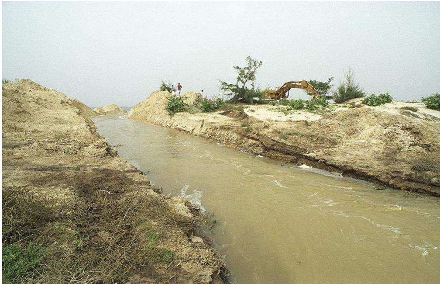
Fig. 2. October 2003: breaching Barbarie spit. Mechanical digger in the background, looking west. (Photo: M. Gerrer, handed over by N. Guiguen, IRD).
