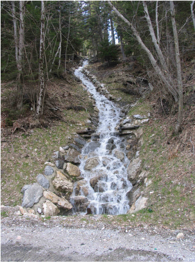
Fig. 11. Detail of the surface dewatering system on the stable grounds above the panoramic road – channel with a longitudinal slope of around 30%, protected with rip rap.
