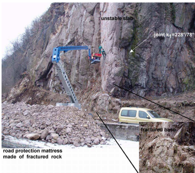
Fig. 7. Detail of the unstable slab and of the fractured rock portion at its base.
