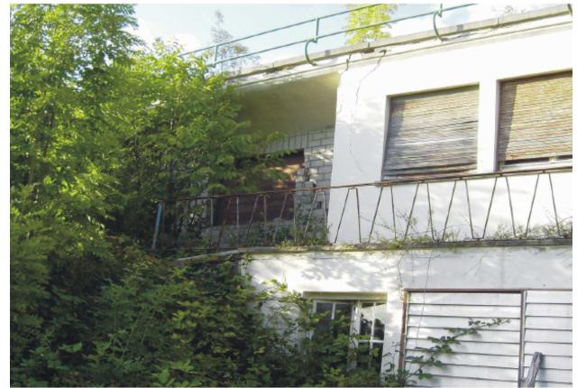
Fig. 2. Residential house in Reutlingen (Swabian Alb) damaged by a landslide (Blöchl and Braun, 2005).
