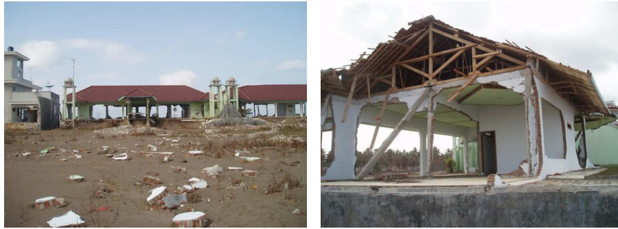
Fig. 13. Two relatively well-made apartment complexes (a) with rudimentary reinforced concrete columns (b), after inundation to a depth of 3.8 m.
