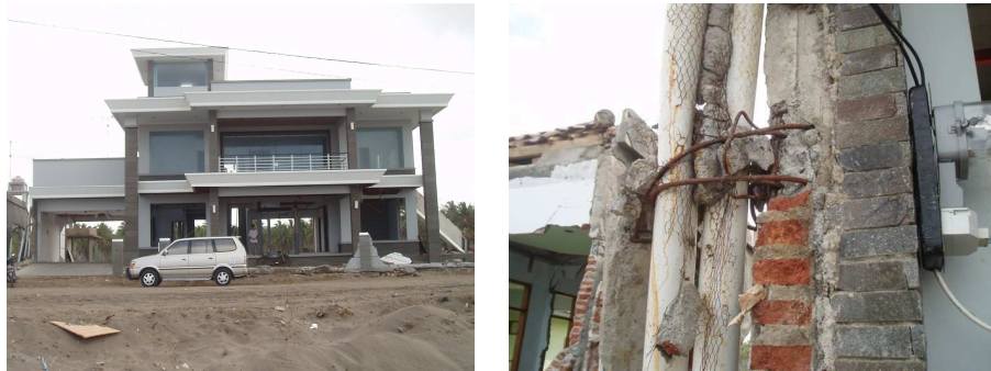
Fig. 14. Well engineered beachfront villa after inundation to a depth of 3.8 m (a). Reinforcement detail is shown at right (b).
