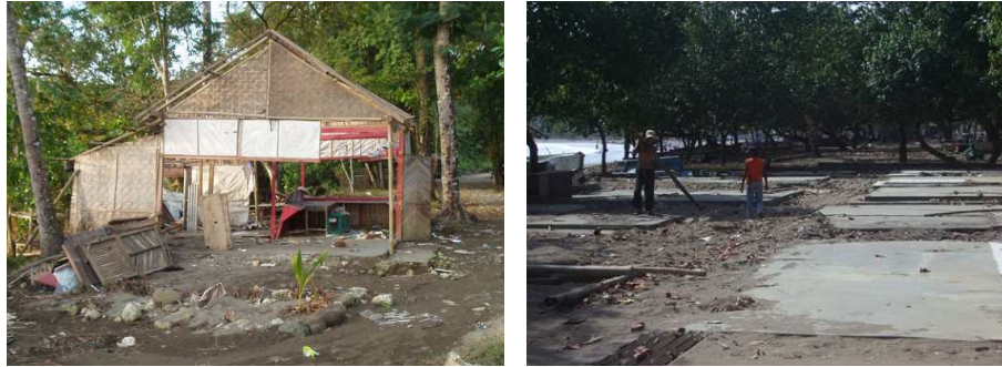
Fig. 11. Typical damage to semi-permanent wooden shops, after inundation to nearly 1 m depth (a) and to 3 m (b). Only the concrete floors remain in the right image, where prior to the tsunami there had been a row of more than 30 shops.
