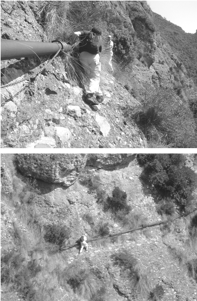
Fig. 9. The Caselle aqueduct trail (also known as “via dei Tubi”) is one of the most hazardous trails in the western sector of Portofino Park.
