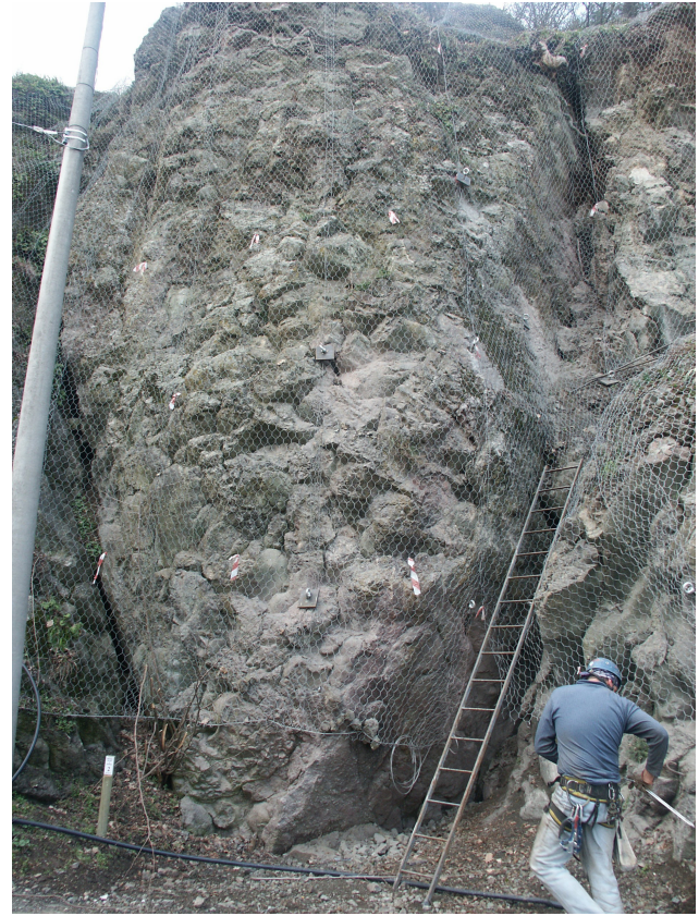
Fig. 6. Unstable basaltic block at the base of the cliff.
