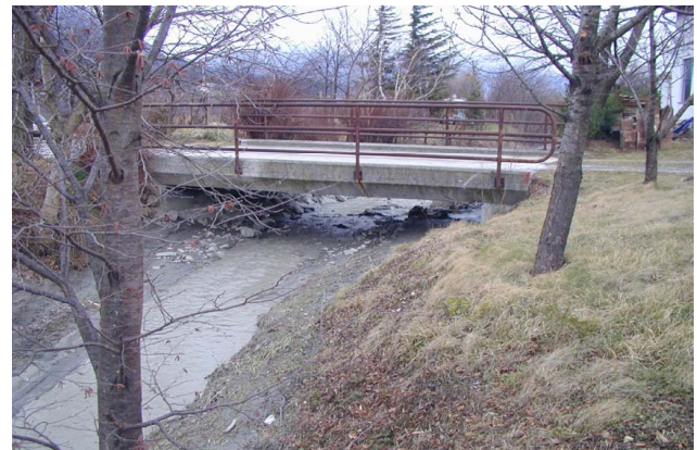
Fig. 21. The area of Grajšček stream cross-section under the bridge is important for the flood and mudflow safety and therefore needs constant maintenance. The photo shows the cross-section partly filled with mud, which needs intervention.
