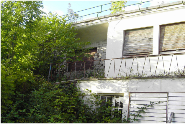
Fig. 6. House damaged by a landslide in Reutlingen. The photograph shows cracks between the main building and an extension.
