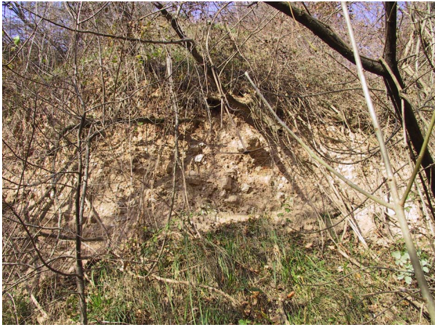
Fig. 9. Banks instabilities along the channel (tract 3). Sub-vertical banks with instabilities related to erosive processes are evident.
