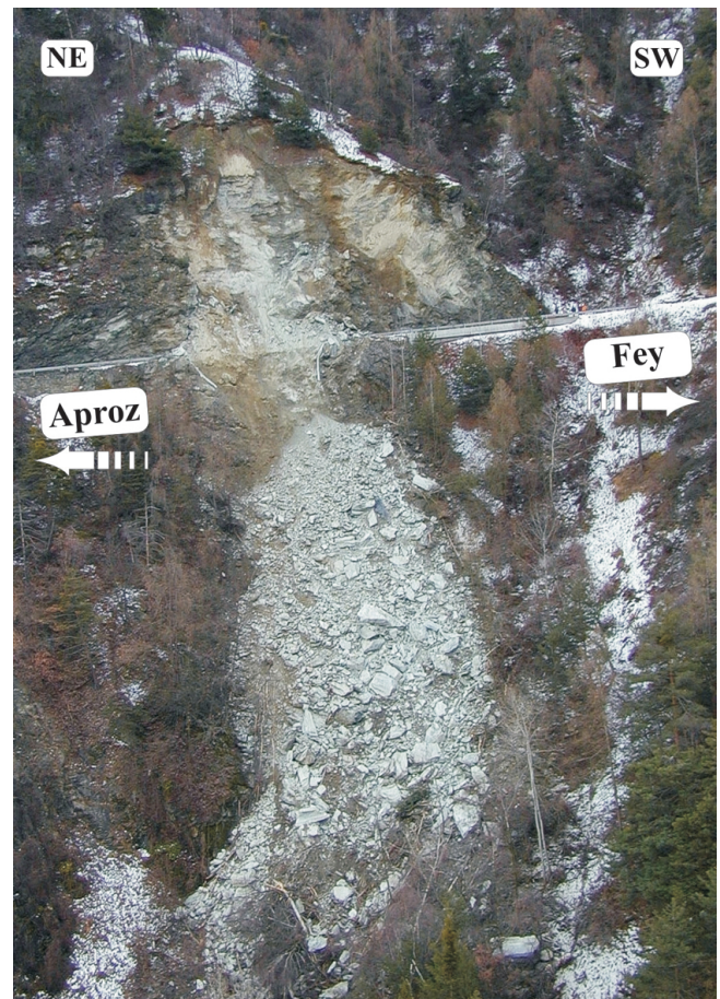
Fig. 2. The Eterpas area after the 9 January 2001, rockfall (photo J.-D. Rouiller). The 30-m-high sub-vertical rock cliff overhanging the road collapsed at 17:30, blocking the road.
