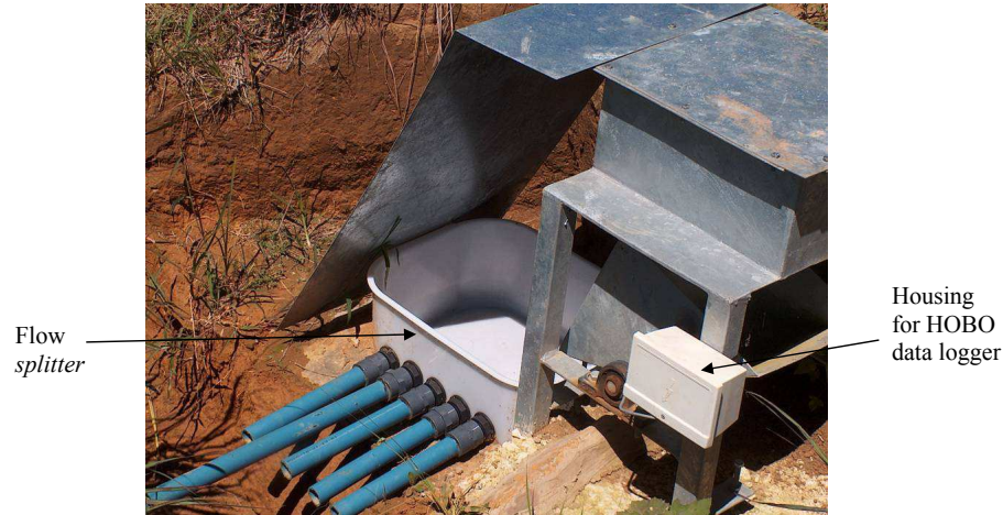
Fig. 7. A flow splitter attached to a tipping bucket, showing the five outlet pipes, only one of which drains to the sample tank.
