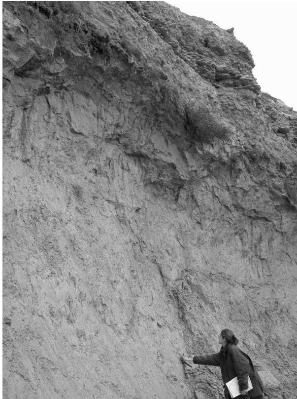
Fig. 9. Exsurgence to the sea along the cliff near Cerano of the aquifer formed by the Pleistocene marine Terraced Deposits overlying the Pleistocene clays.
