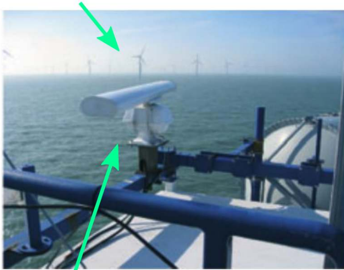
Offshore wind farm (Horns Rev, Denmark)
